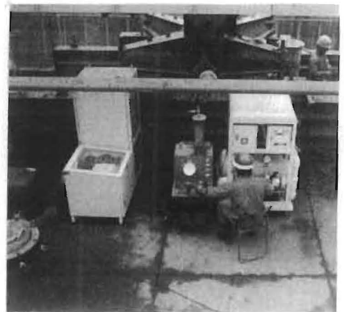
Fig. 12 Controllers on the top slab
