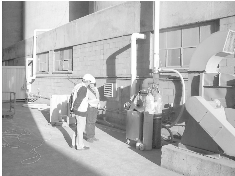
Figure 4. The HDS-80 connection with the cylinders of nitrogen and VAPORPH 3 OS.
