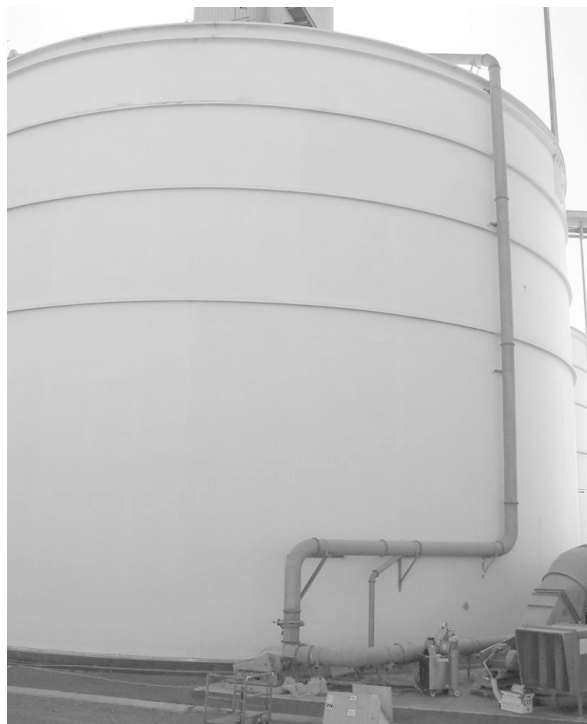
Figure 5. The 10,000-tonne welded steel sealed silo with the HDS-80.
