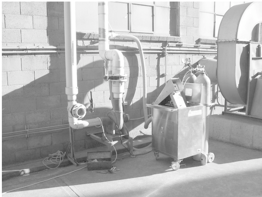
Figure 3. The HDS-80 and flexible hose connections to the phosphine/air inlet and recycling air outlet downstream of the recirculation fan.
