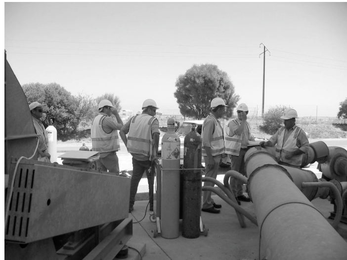
Figure 7. Flexible hose connections to the recirculation duct of the 10,000-tonne silo.
