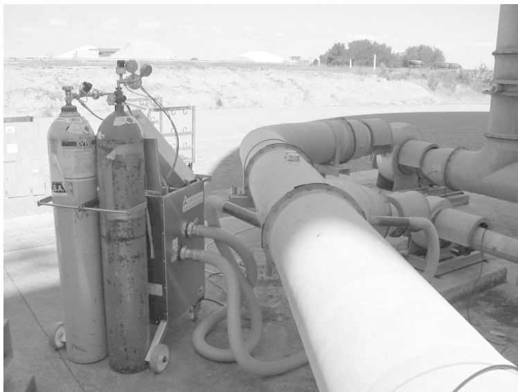
Figure 8. The HDS setup and the two fans, the bigger 7-kW methyl bromide fan and the smaller 1.5-kW phosphine fan.
