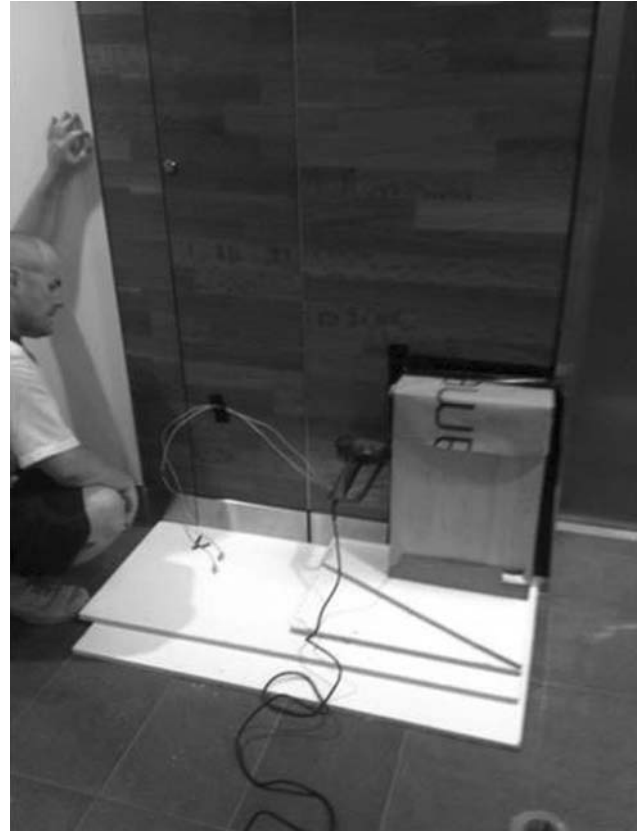
Fig. 5. Small plenum and heat gun in place for retreatment of infestation surviving first treatment series
