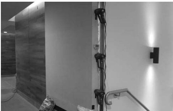
Fig. 4. Heating enclosure (plenum) in place on Panel 16, First floor, showing installed heat guns and datalogger
